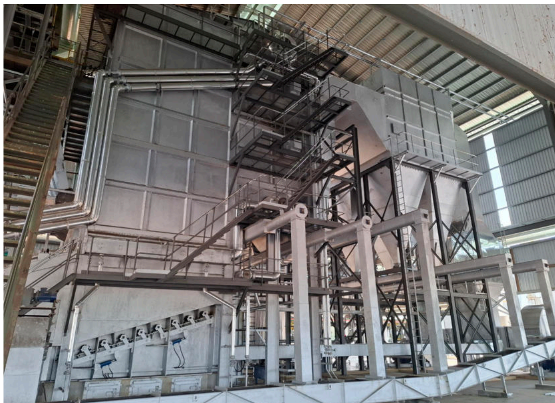
Cha Uat Boiler Station
