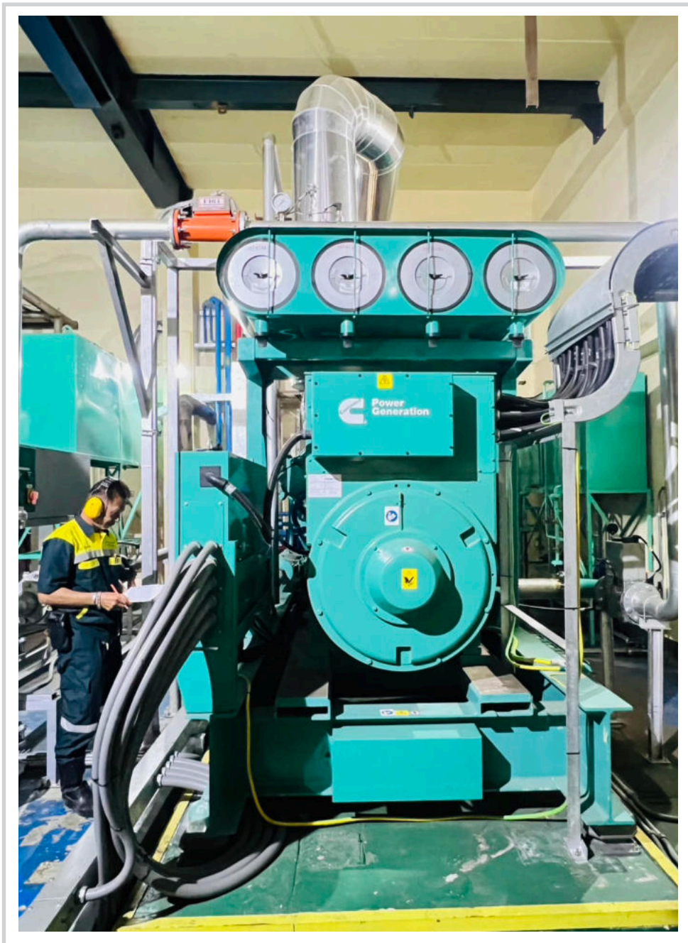
Topi Replacement Gas Engine
